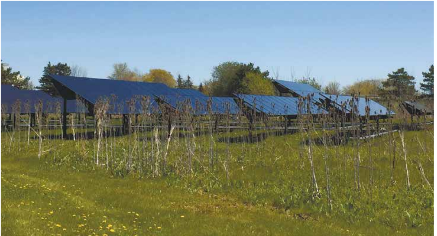
Solar Station at the University of Buffalo
