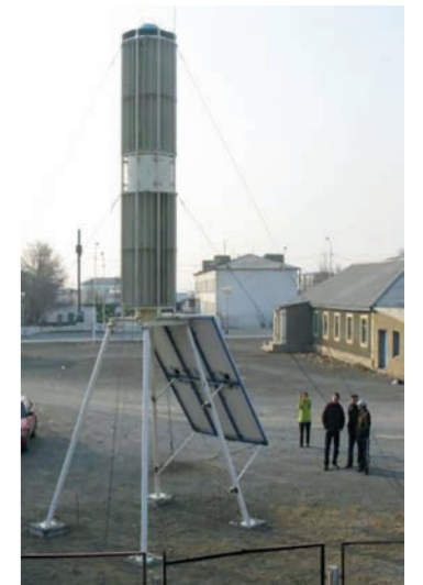
2006, CPP VRTB -2.6 on the site of Kazakhtelecom JSC, Azhar settlement, simultaneously supplies power to the electronic equipment of the school, and the Internet.
