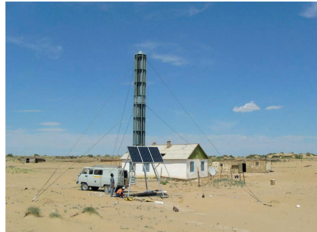
1996. Installation of solar-wind plant to supply power to facility of Kozhakazgan settlement, Kyzylorda region. The customer is Kazakhtelecom JSC.
