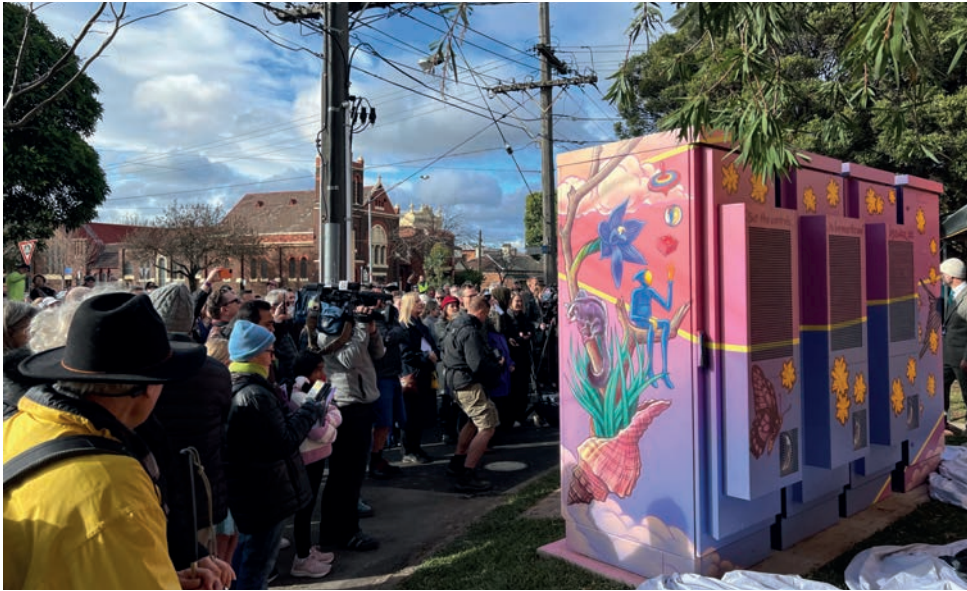
Neighborhood battery in Victoria, Australia
